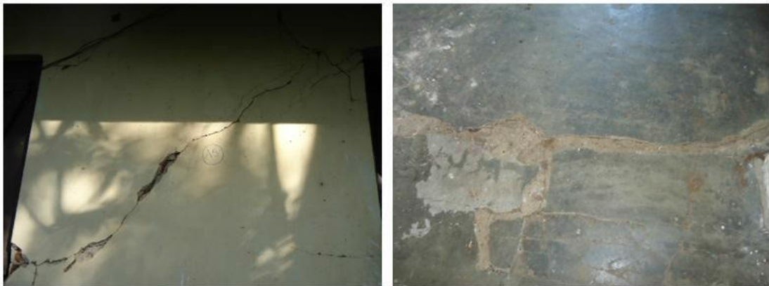
(a) Wall cracks
